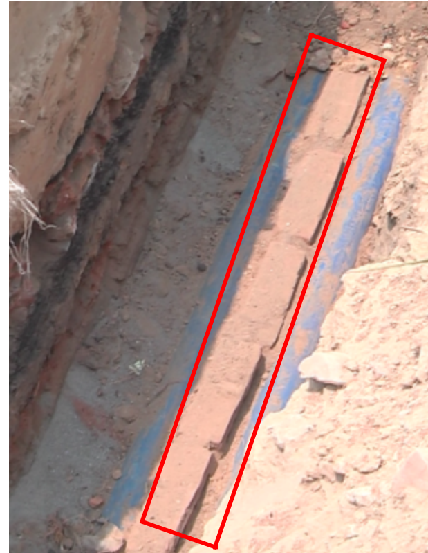
Circuits running parallel with brick padding
