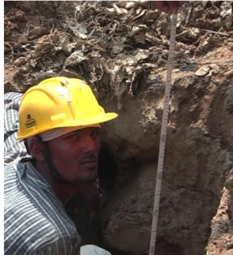
Depth of the pit is more than one metre
