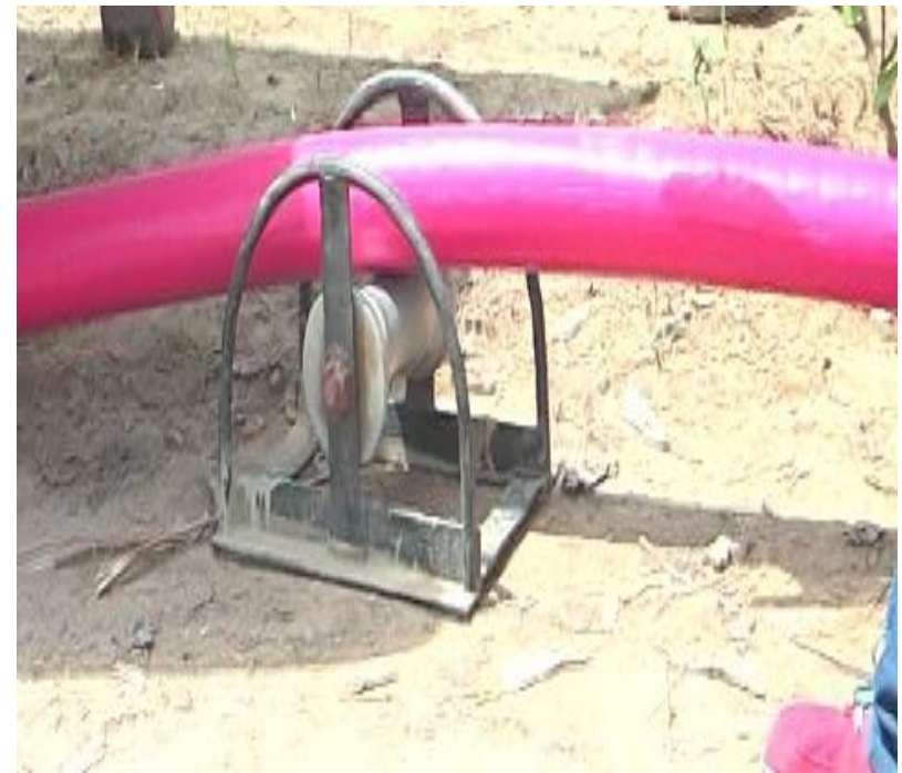
Rollers through which the cable passes
